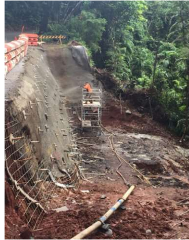
First stage of repairs saw large soil nails drilled into the hard rock underneath
