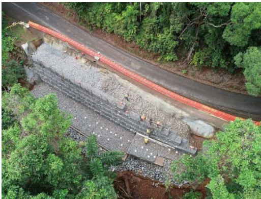
Contractors have been drilling specialised soil nails and spraying it with concrete to keep the area secure
