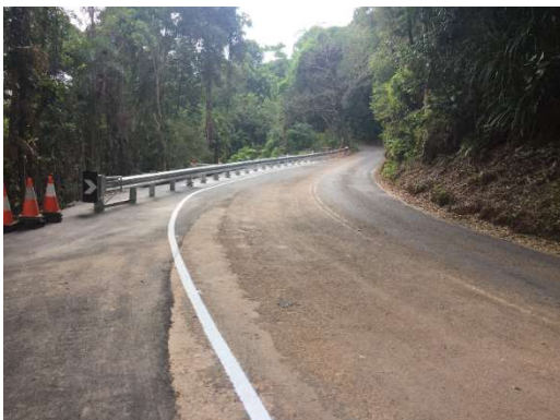
The Alexandra Range Landslip has been rehabilitated and the Cape Tribulation Road reopened to normal conditions 11 September 2019
