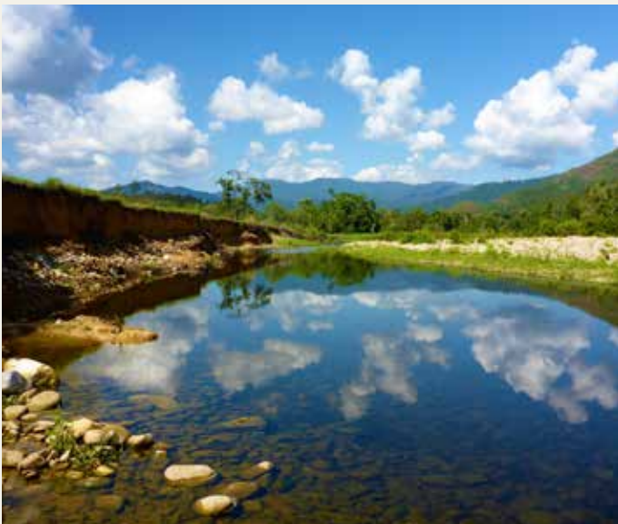
Streambank erosion following STC Debbie – site SH7 at St Helen’s Creek. Source: Neilly Group Engineering
