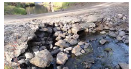
Provide close up photos supporting damage to all damaged asset components – eg upstream, downstream and approaches
