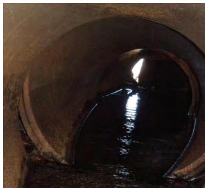
Demonstrate the nature and full extent of event damage to asset components. E.g. inside damaged pipe showing damage
