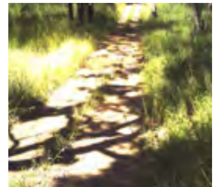
Cannot make out damage to asset due to shadows
