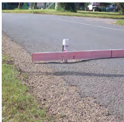
Use of straight edge, taken close up and angled level with the damage
