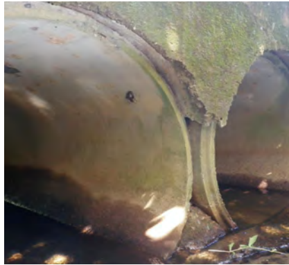
Demonstrate event damage to claimed asset components
