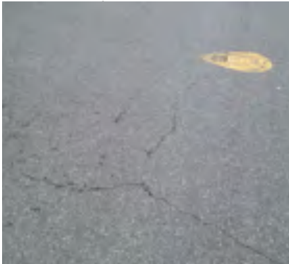
Location, nature and extent of damage to an eligible asset is not evidenced. No asset visible, no significant damage directly related to an event, no perspective of the scale of defects or location.
