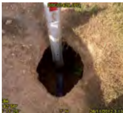
Use of post or measure to demonstrate depth of subsidence
