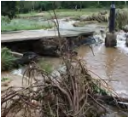
Provide a visual perspective of the nature and extent of damage to the asset and damaged components
