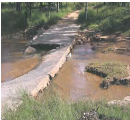
Show surface and structural damage to asset and approaches
