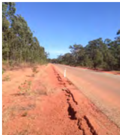
Photo demonstrates location nature and extent of event damage to the asset
