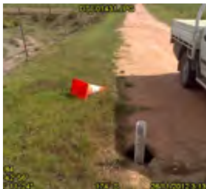
Use a measure, ruler or other available prop to demonstrate extent and nature of damage and support proposed scope of works – e.g. sinkholes/blowholes
