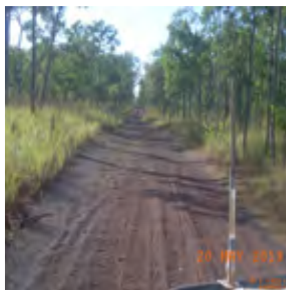
Evidence supporting nature and extent of asset damage is consistent along the distance
