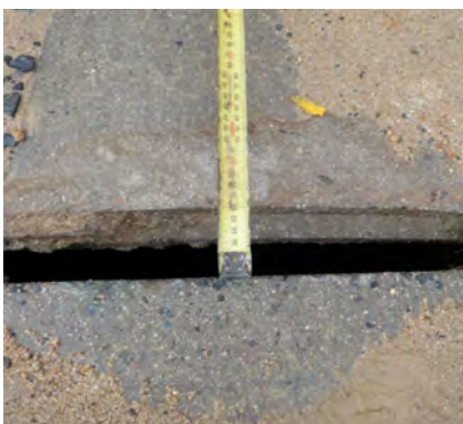
Use a tape to demonstrate the extent of damage to pipe
