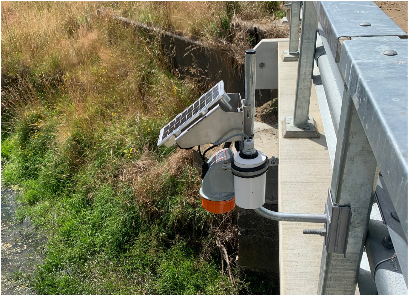
Radar water level sensor coupled with a battery-powered data logger and solar panel (Credit: Horizons Regional Council and Metasphere)
