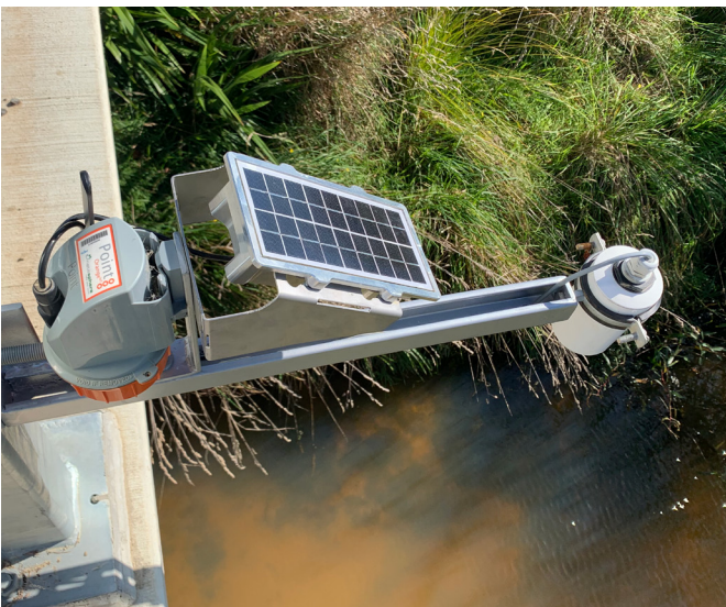
Radar water level sensor coupled with a battery-powered data logger and solar panel (Credit: Horizons Regional Council and MetaspHERE)
