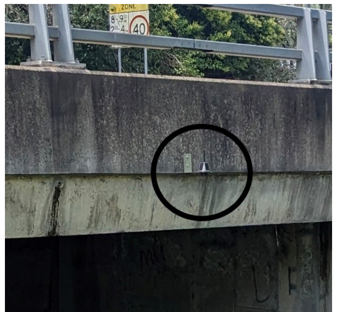
Radar water level sensor and data logger (Credit: Ontoto)
