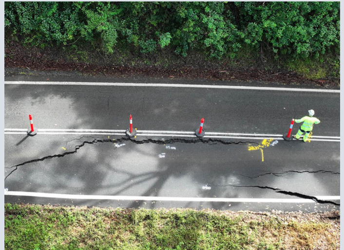
Beechmont Road – initial cracks signalling embankment failure after SEQ Rainfall and Flooding (early March 2022)
