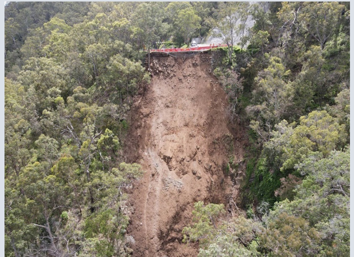
Lamington National Park Road – major landslide site (December 2021)
