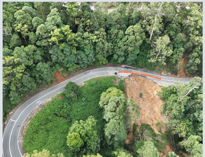
Beechmont Road – embankment failure (late March 2022)
