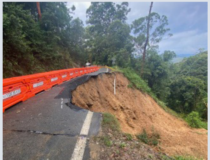
Beechmont Road – embankment failure (late March 2022)
