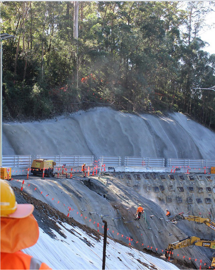
Beechmont Road – embankment failure (late March 2022)
