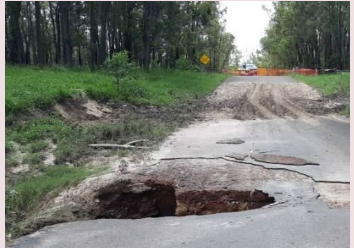
Culvert damage at Gwambegwine Creek (Dec 2021)
