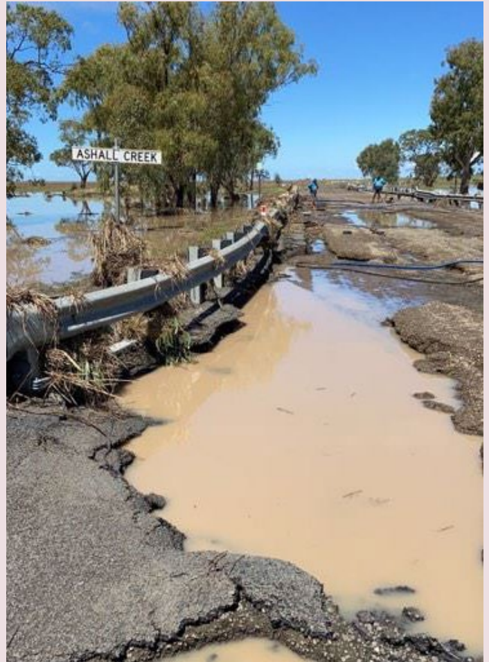
Damage from SEQ Rainfall and Flooding (April 2022)
