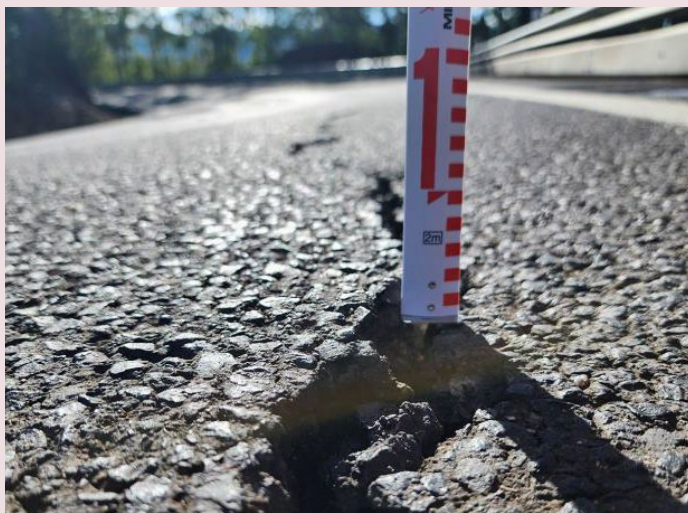
Pavement cracks (May 2024)
