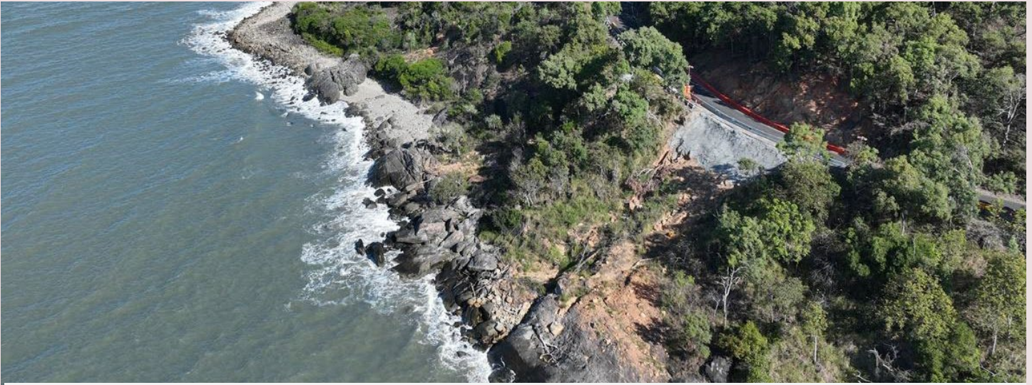
Captain Cook Highway – major landslide site (September 2024)
