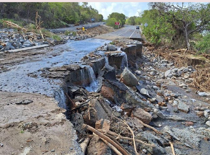
The destruction from Jasper closed roads and isolated communities
