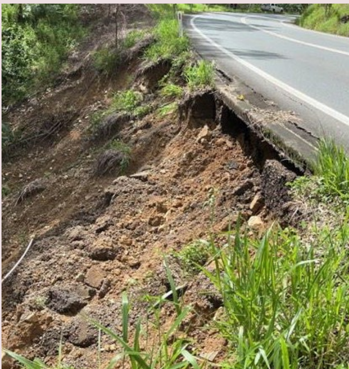
Landslip caused by SEQ Rainfall and Flooding event (March 2022)
