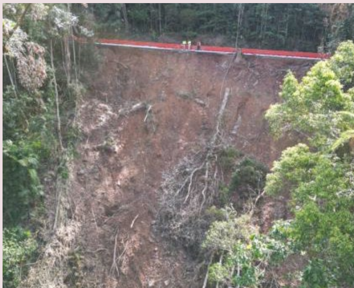
Massive landslips on Alexander Range Road made it unsafe for traffic
