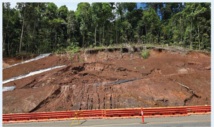
Palmerston Highway – major landslip site 2 (February 2024)
