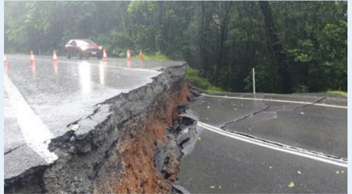
Palmerston Highway – major damage from TC Jasper at site 1 (December 2023)
